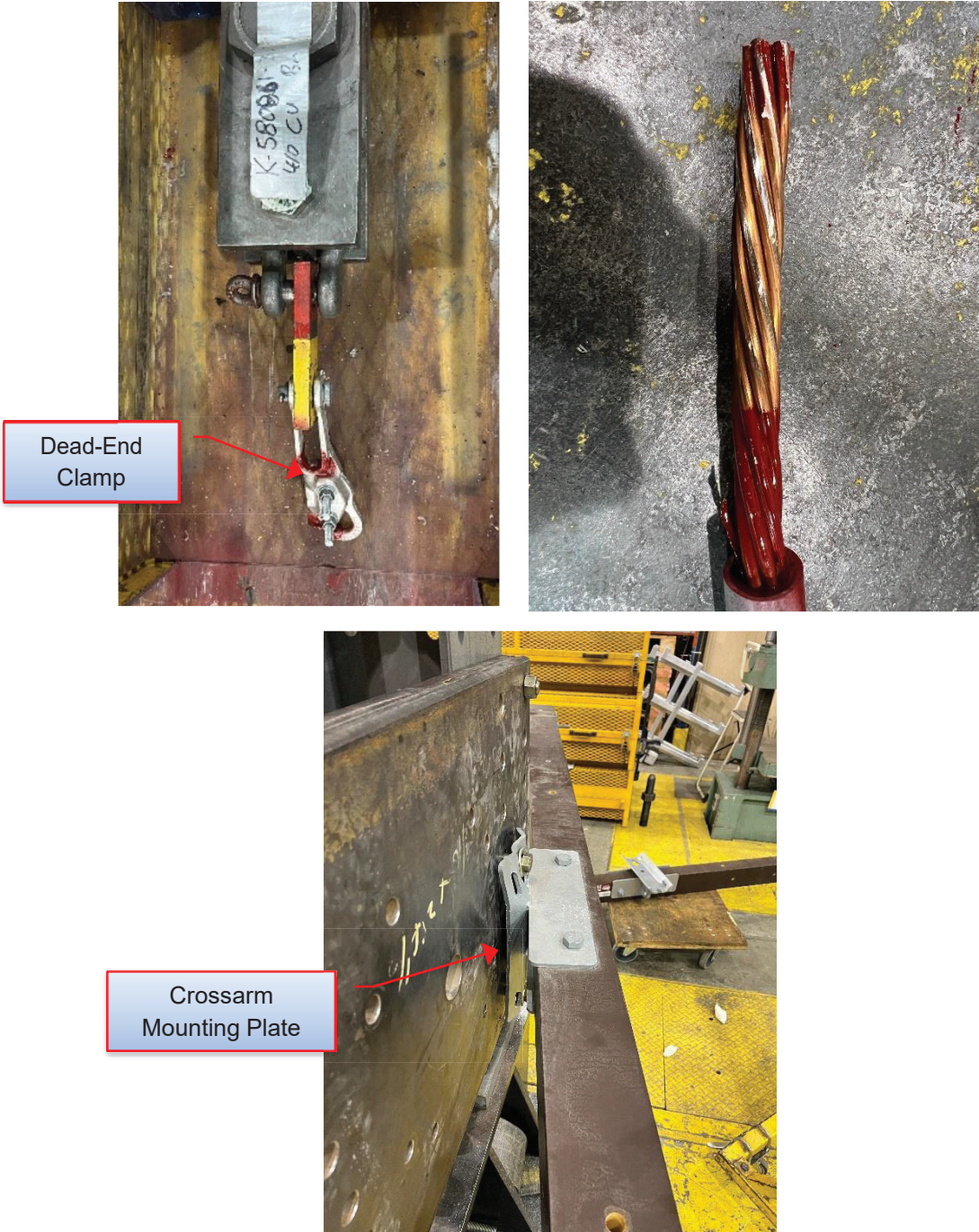
Figure 6-16: Sample 3.3 – Failure Location
