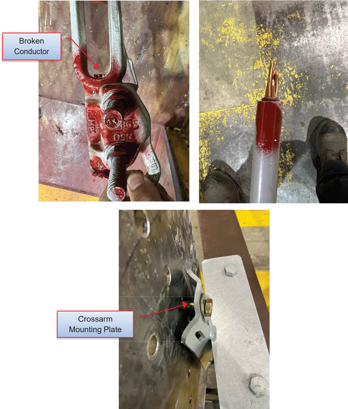
Figure 6-8: Sample 1.1 – Failure Location
