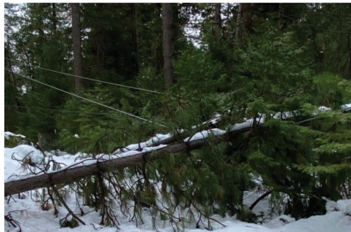
Figure 4: PG&E Covered Conductor Effectiveness – Example 3
