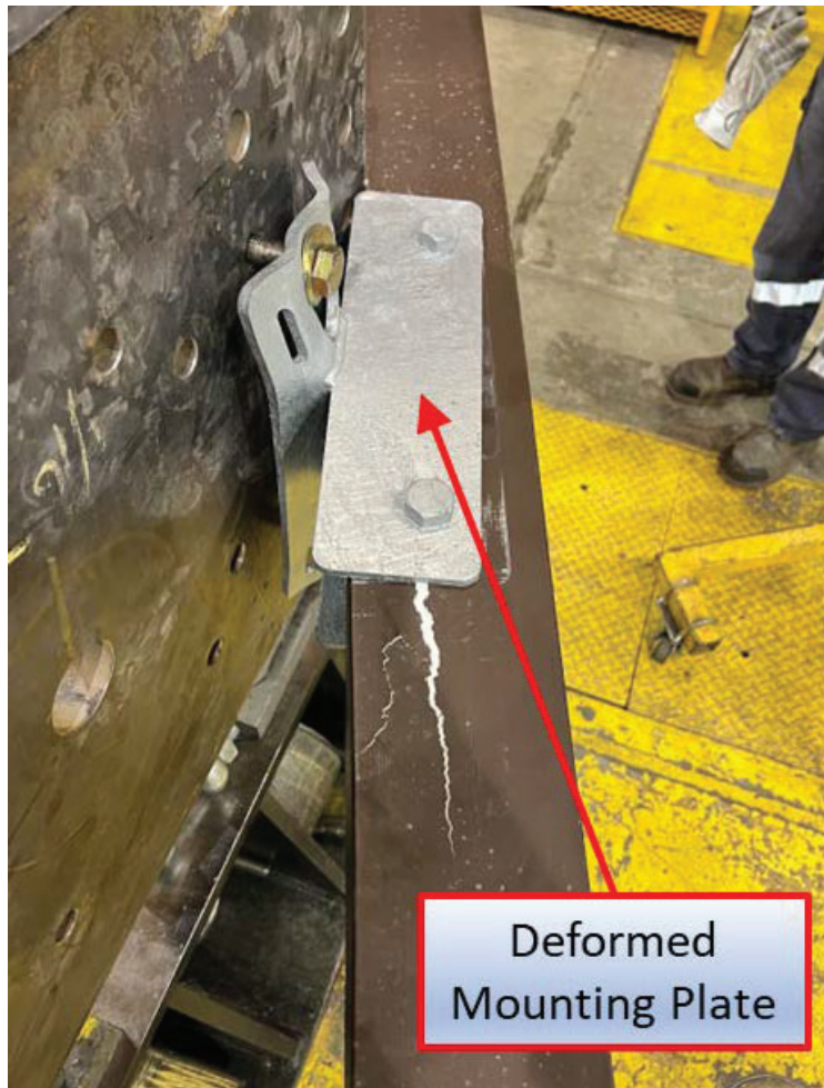
Figure E5. A representative post-test image showing typical deformation of the cross-arm mounting plate.
