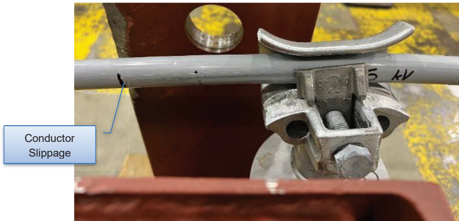
Figure 6-10: [REDACTED] - Typical 1/0 AWG ACSR (35 kV) Conductor Condition after Slip Test
