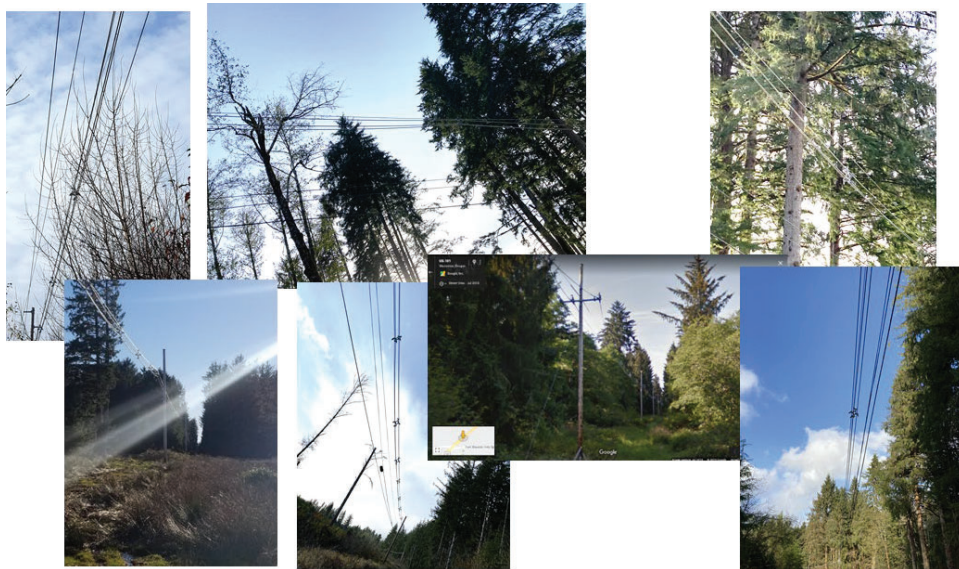
Figure 5: PacifiCorp Covered Conductor Effectiveness Examples
