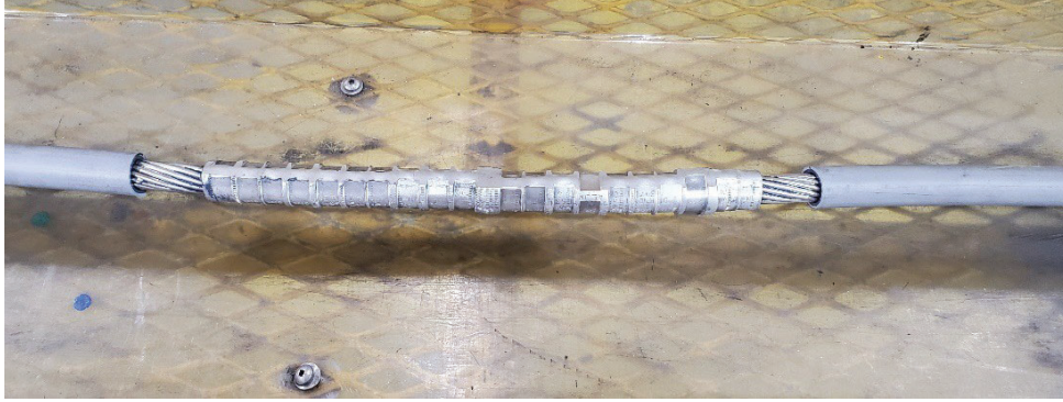
Figure 3-4: [REDACTED] Installed on 22 kV 397.5 kcmil, 19 strands AAC
