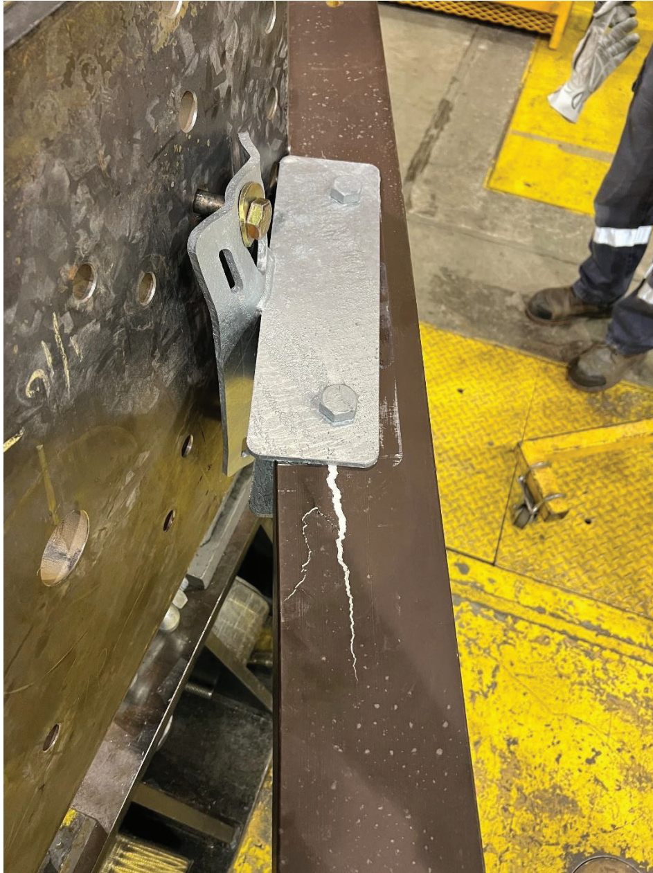
Figure 6-17: Sample 4.1 – Failure Location
