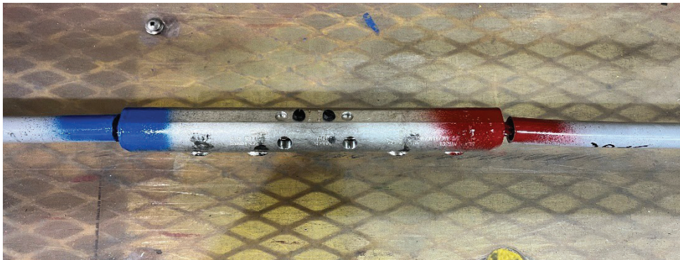
Figure 3-5: [REDACTED] Installed on 15 kV 1/0 AWG, 6/1 ACSR
