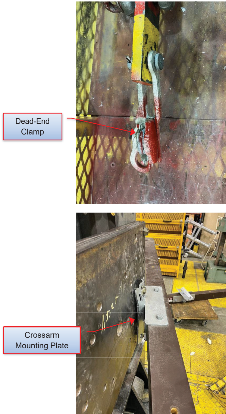
Figure 6-15: Sample 3.2 – Failure Location
