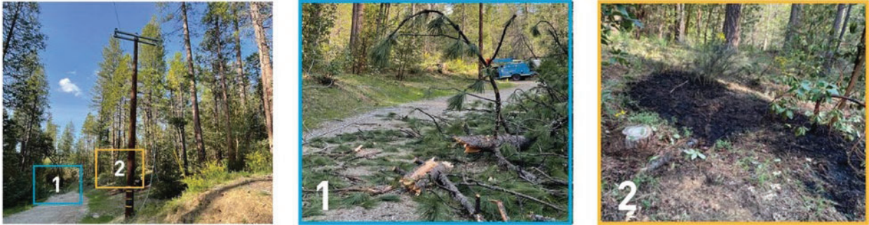
Figure 3: PG&E Covered Conductor Effectiveness – Example 2
