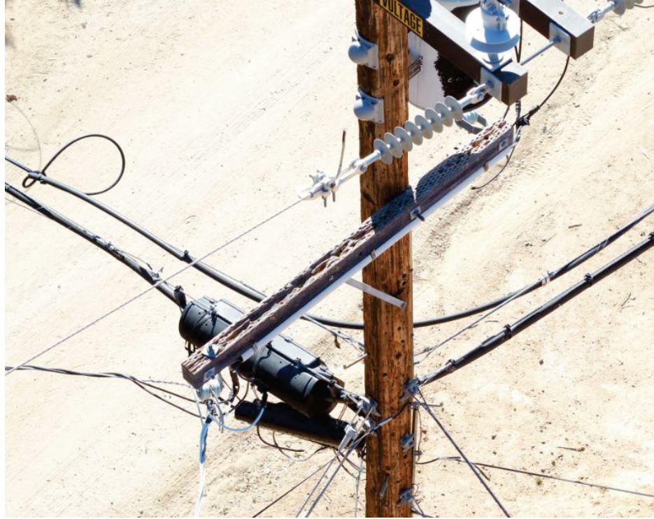
Figure JW-9 Crossarm damage only visible from above
