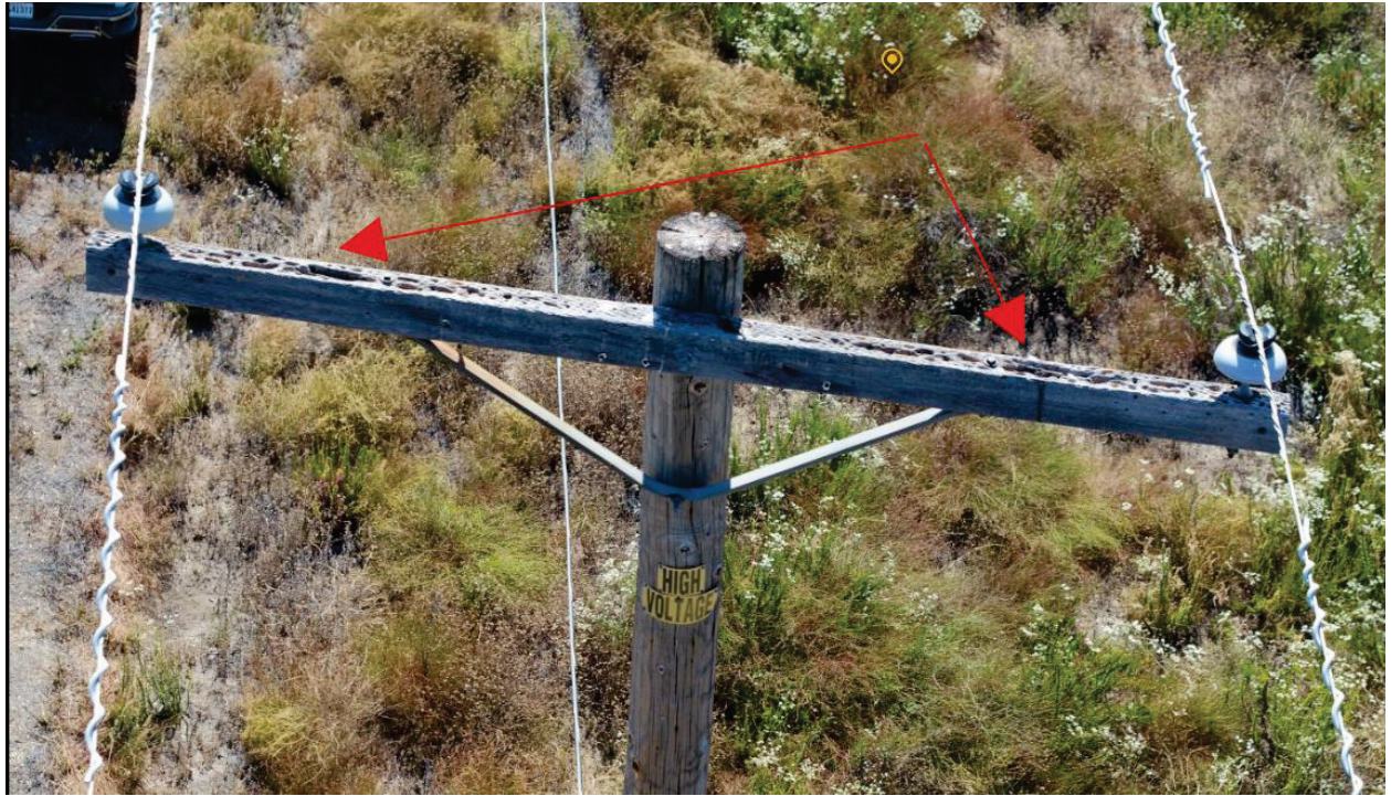
Figure JW-13 Crossarm damage only visible from above
