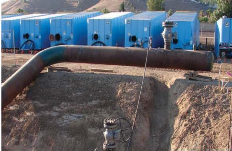
Figure 26: Water Tanks and Test Head
